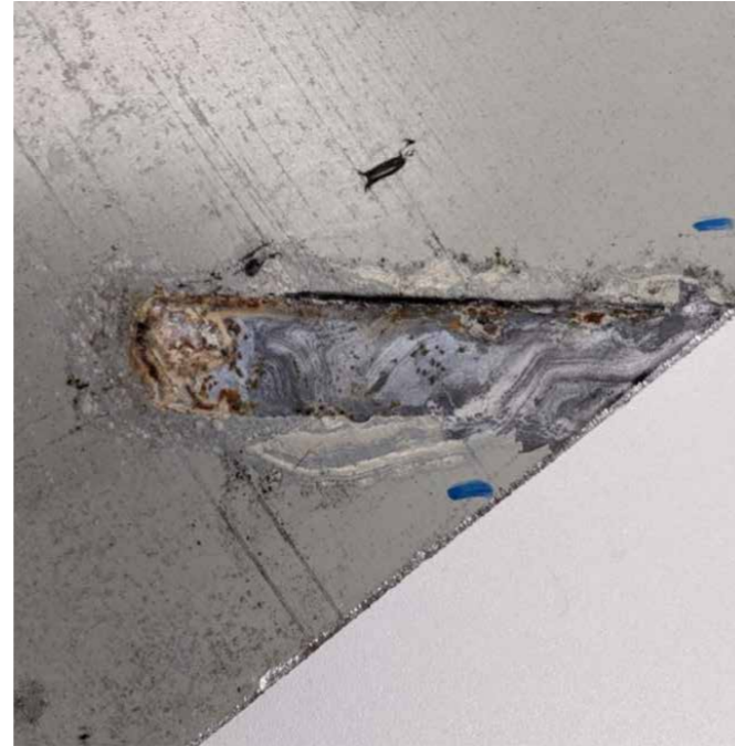
Figure 2: Galvanic corrosion observed around the adhesive bond. The adhesive was not insulating enough and allowed the two dissimilar metals to transfer charge, causing galvanic corrosion.
